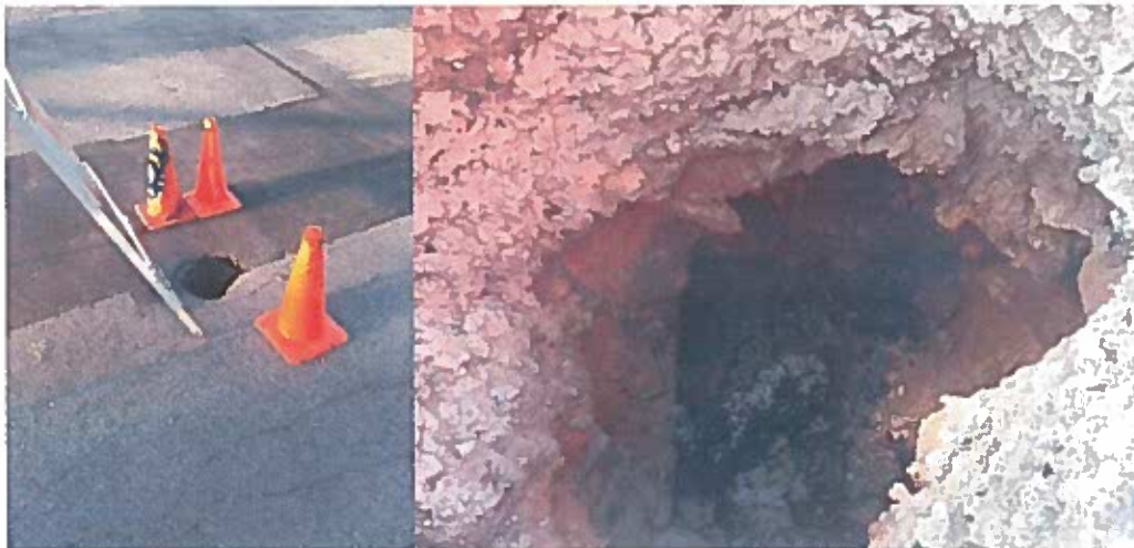
Neville Parking Lot Sink Hole: discovered Friday, June 2, 2017, excavated and filled Thursday, June 8, 2017. Water was trapped in the basement foundation of the former Blackstone Restaurant. Water was pumped out and fill was replaced in the cavity.
