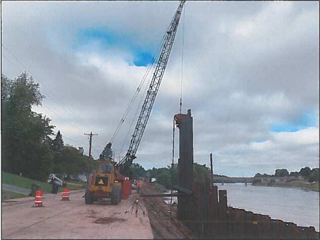
CTH ZZ – McMullen & Pitz and Vinton Construction installing new sheet pile wall and tie-backs as part of the WisDOT let project.
