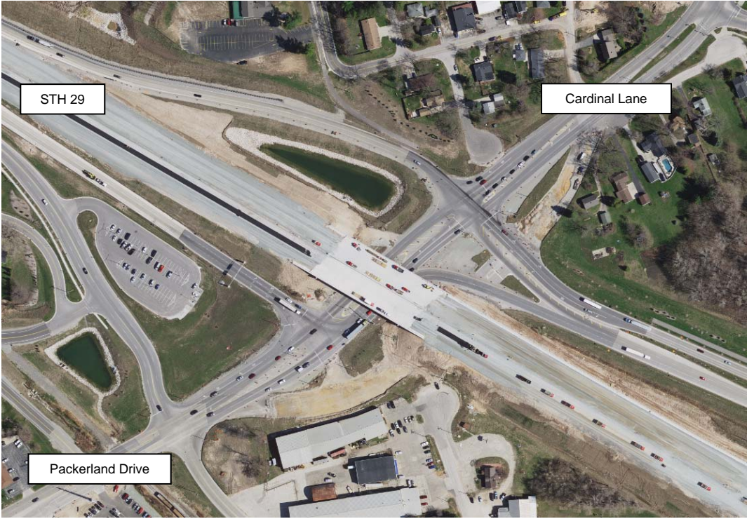
Aerial View of the STH 29 – Packerland Drive/Cardinal Lane Intersection During Reconstruction Project (2014)
