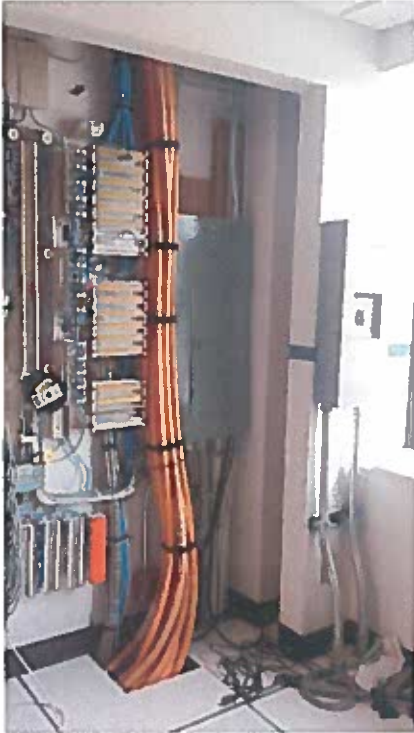
Data Center Fiber and Copper Cabling
