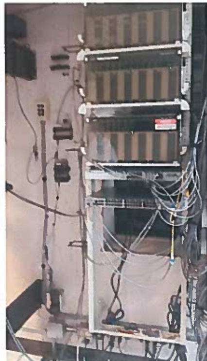
Data Center Copper Cabling
