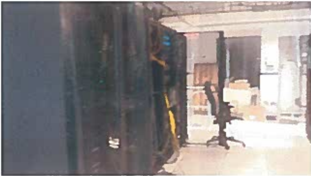
Data Center Racks w/ temp control sheeting
