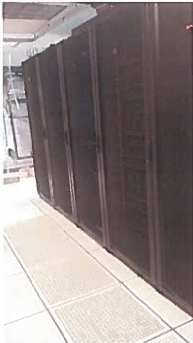
Data Center Racks
