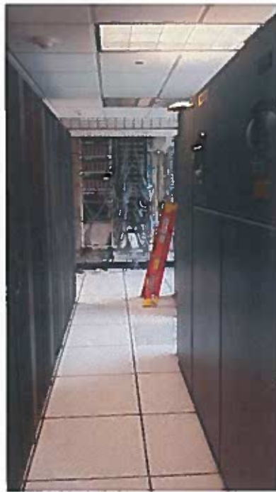
Data Center Racks
