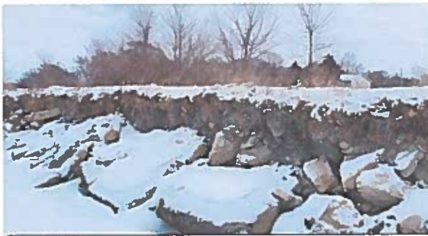
FIGURE 6 COLLAPSED BREAKWATER FACE
