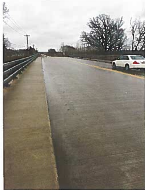
No sign that bike lane ends
