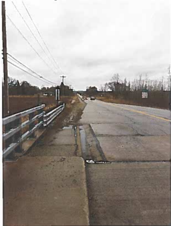
Shoulder is not paved after bridge
