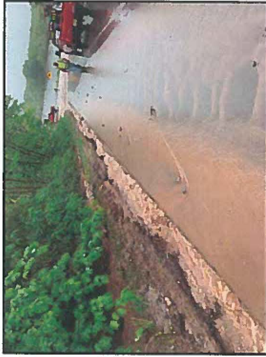
Flooding CTH ZZ, May 2020 Photo credit: Brown County Public Works
